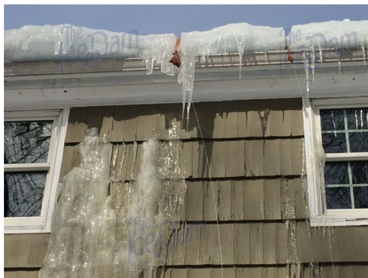
These salt socks didn't melt down to the roof, resulting in massive water damage to the interior walls. (Can you find the ice on the siding?)
